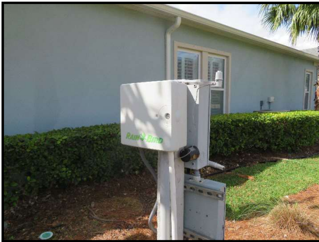
Irrigation system controller
