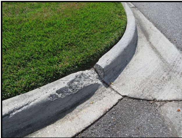
Isolated curb damage
