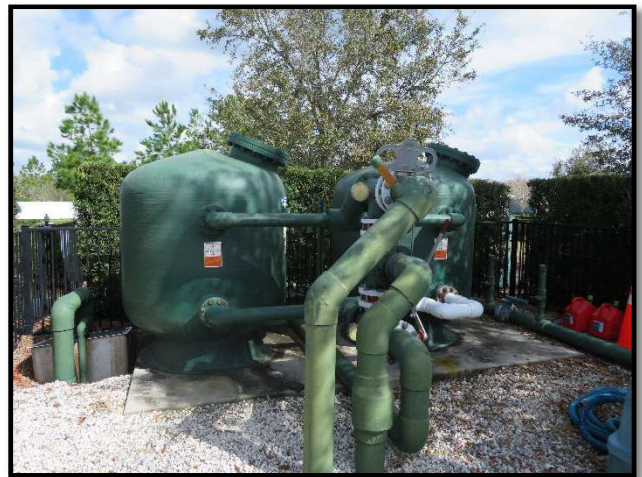
Pool mechanical equipment
