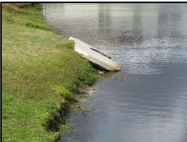
Minor settlement behind pond inlet structure
