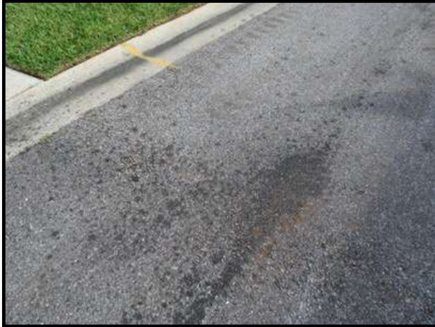
Vehicular fluid stains at alley adjacent to Claymore Street
