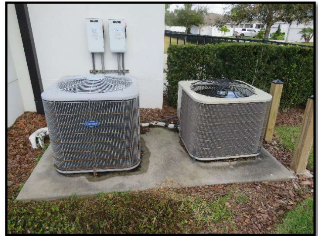
Air condensing units at Fitness Center
