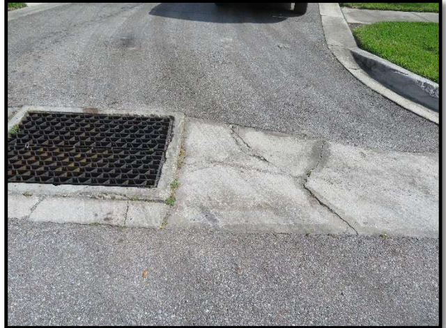
Minor settlement adjacent to catch basin
