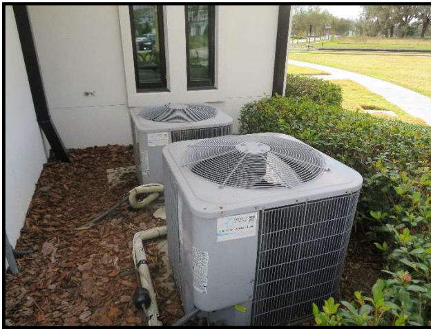
Air condensing units at clubhouse
