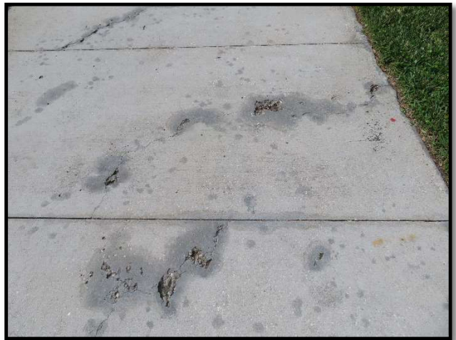
Isolated concrete spalling
