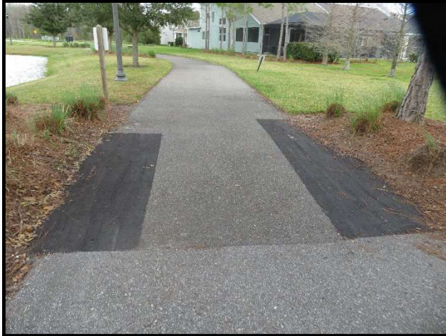
Previous repairs adjacent to boardwalk
