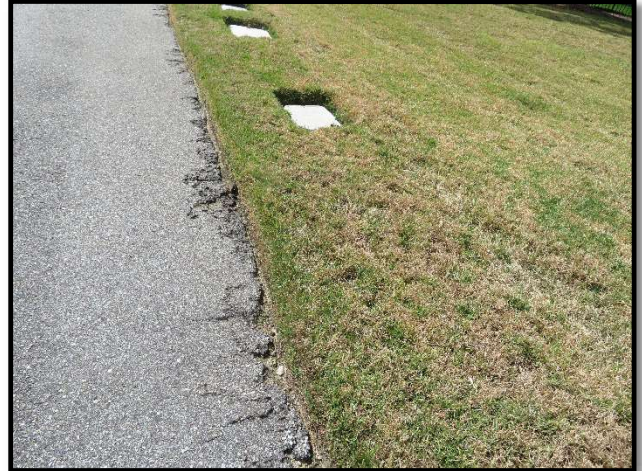
Asphalt pavement walking path edge deterioration
