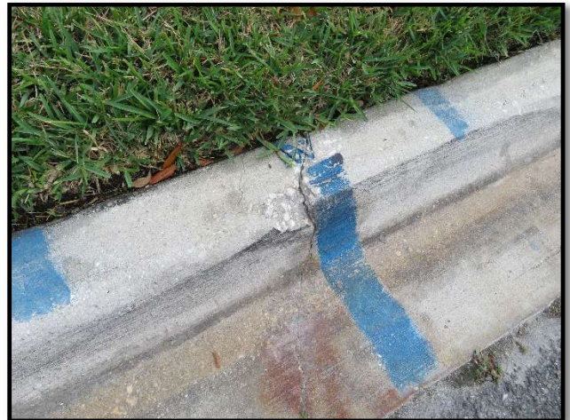
Isolated curb damage
