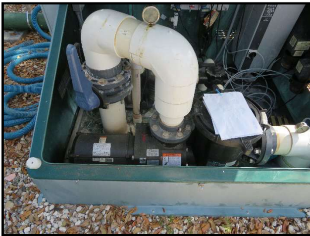
Pool mechanical equipment
