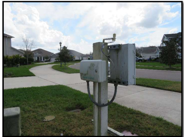
Irrigation system controller
